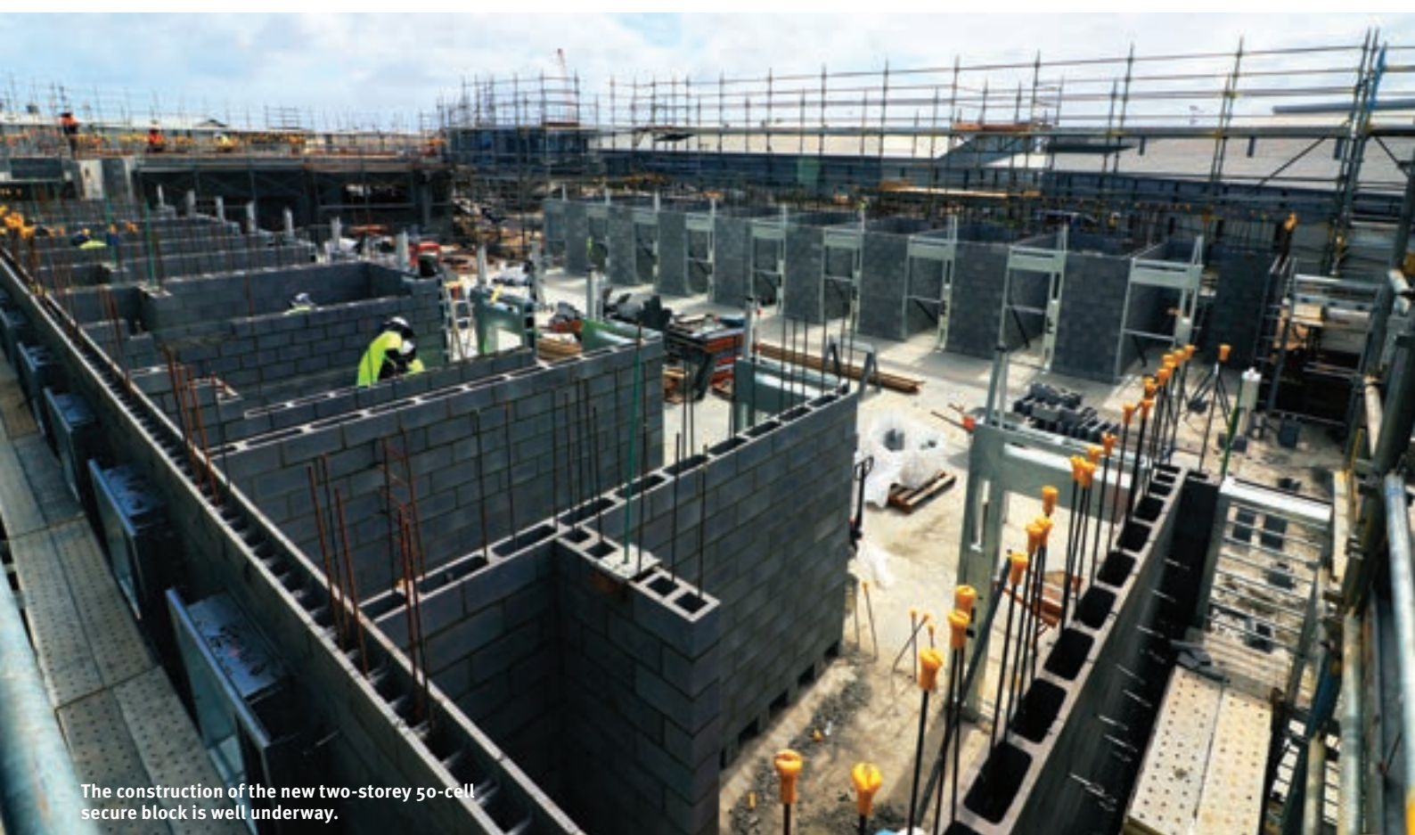
Capricornia expansion Project Director, Shane Hopgood and Deputy Commissioner Koulouris examined the progress so far.
